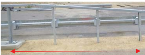
6.3 Feld 1 – Absenkung Handlauf Section 1 – Turned down handrail
