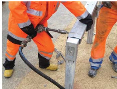
4.15 Bohren des Passstücks an der Endverankerung Drilling of the fitting-piece at the end anchoring
